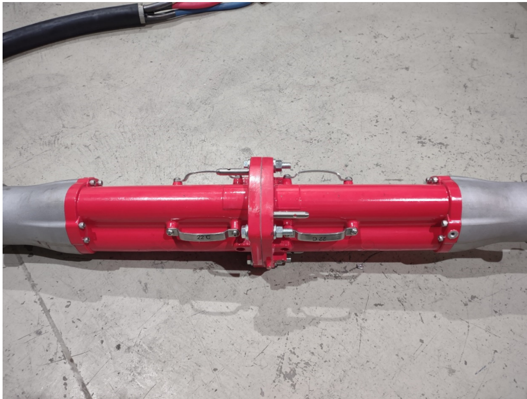
Picture 1 General view of coupler
